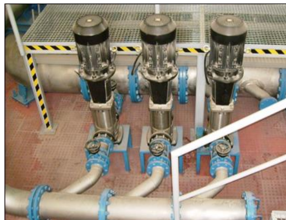
Bombeo 2 San Crispín
